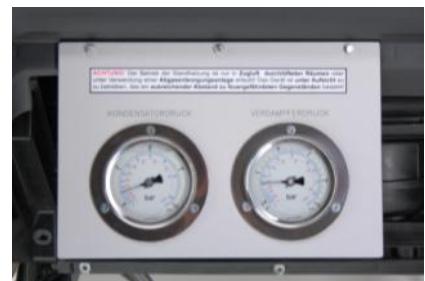
Image shows the indicators for condenser and evaporator pressure
